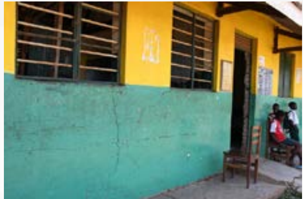
A cracked classroom block at Namilyango primary school which poses a threat to human habitation
